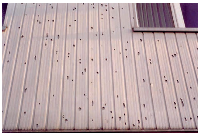
Figure 3: Hail damage in facade made of synthetic material, Wetzikon 2004. (Source: Thomas Egli)
